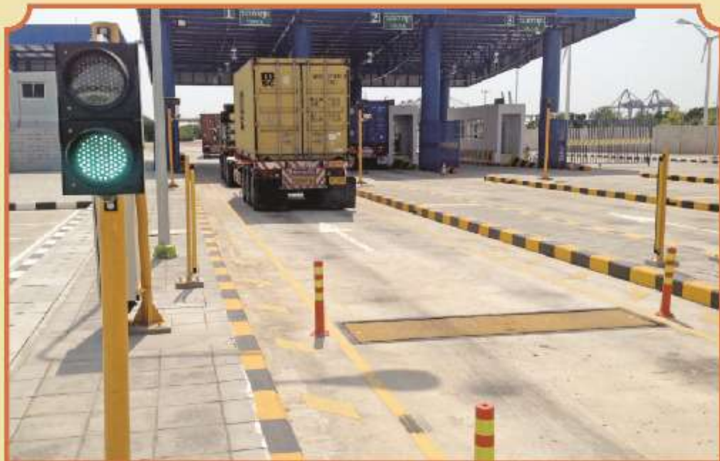
TOLL PLAZA WEIGHING SYSTEM
